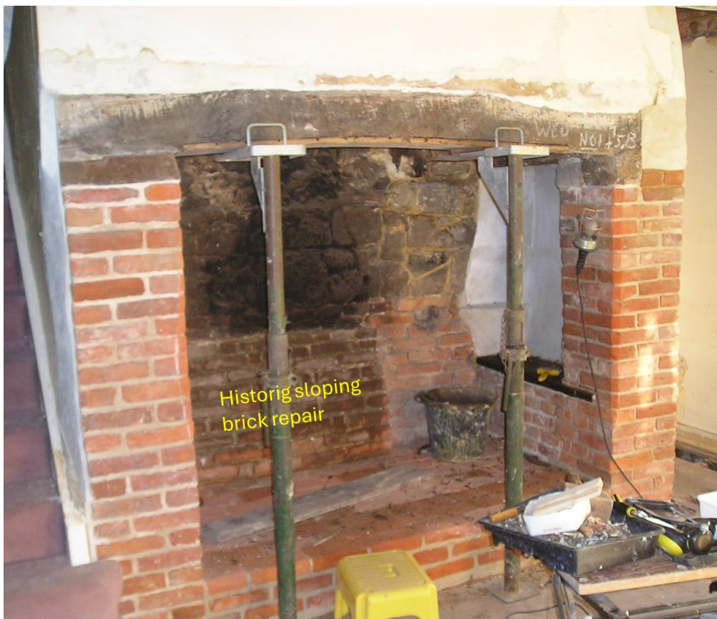
A historic sloping brick repair due to heat damage to a late 16 th century fireplace in Betchworth.
