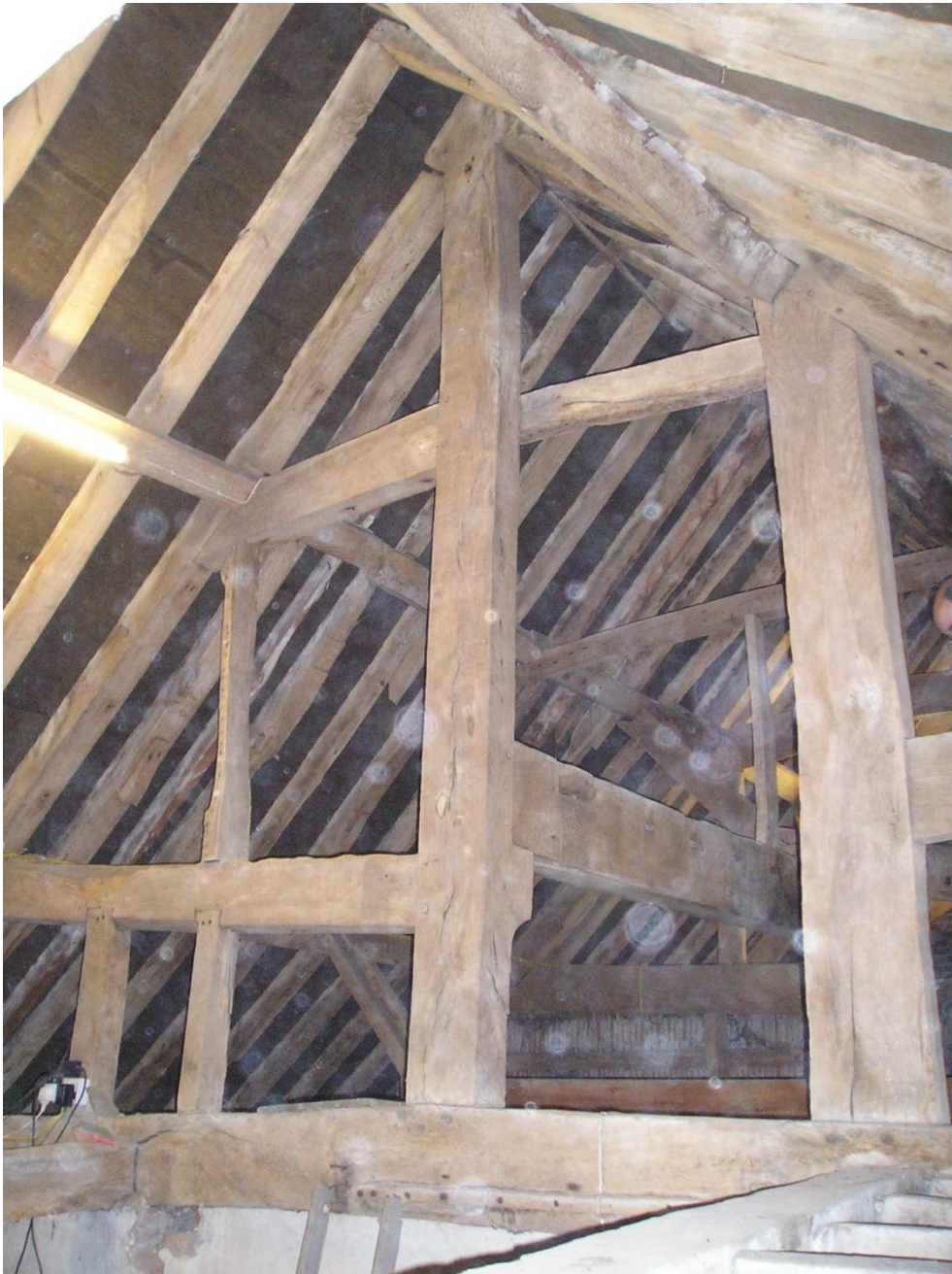
Place Farm, Bletchingley – once the gate house to a Palace. The roof has one of the earliest dated king posts in the country (1547)
