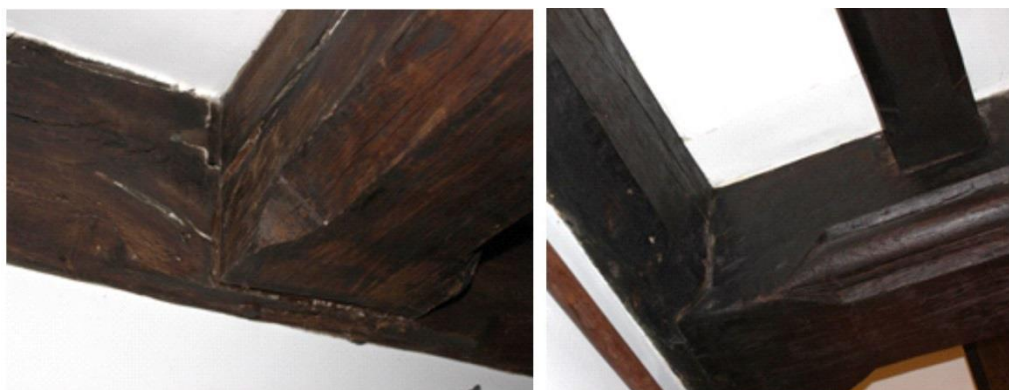
Intersection of axial beams with mid-ties, left image is north side of B, right image is south side C.
