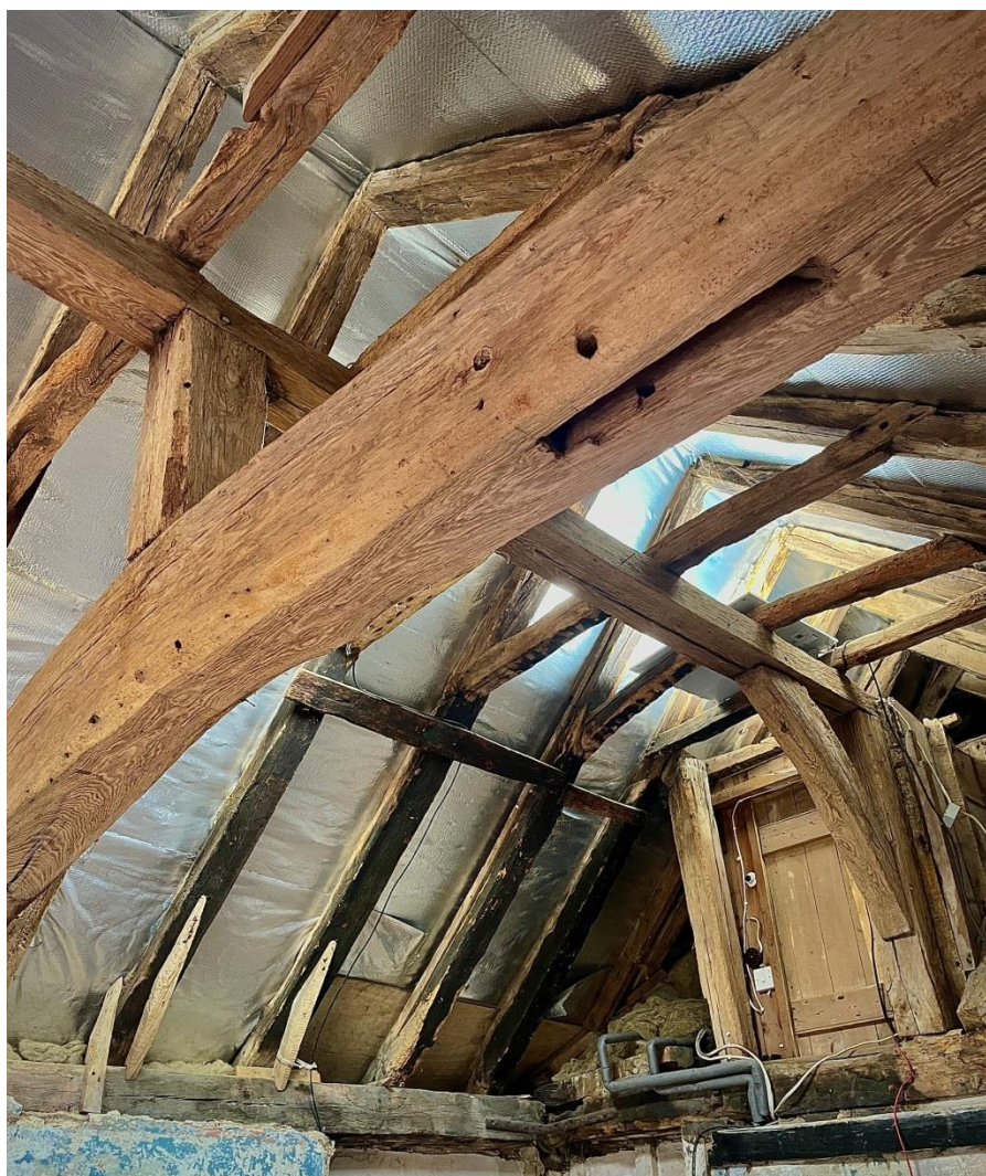
Newly exposed roof structure of Range B, showing smoke blackening in one bay.
